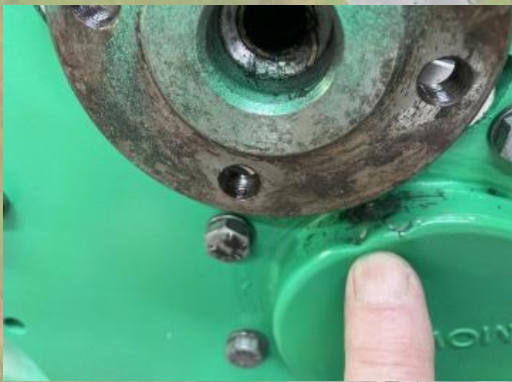
Modified pump can
